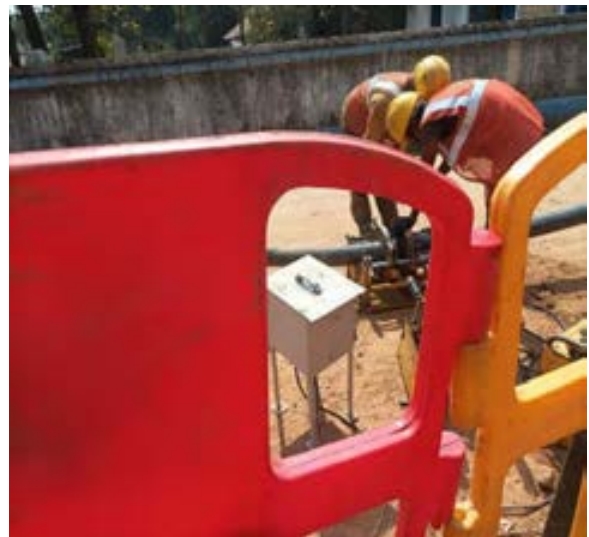
After: Recommend compliance done (Package BK/02B)
