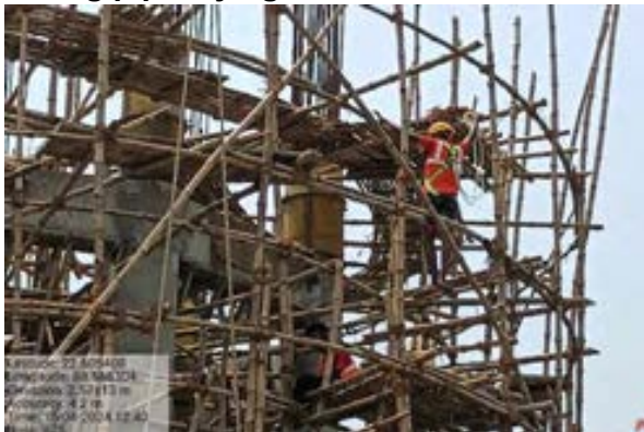
Fig: Zone 5 OHR – Use of safety belt and PPEs when work at height-Bhangar-II Block
