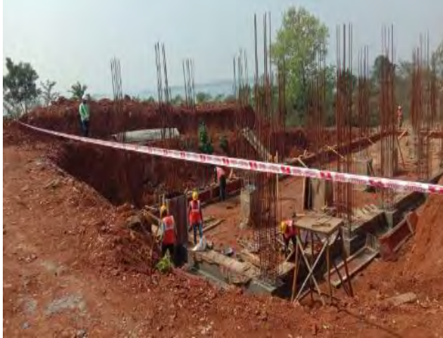
Use of caution tape and Safety signage at WTP site BK/01
