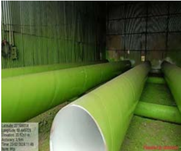
Fig: Spray painting without proper flooring
