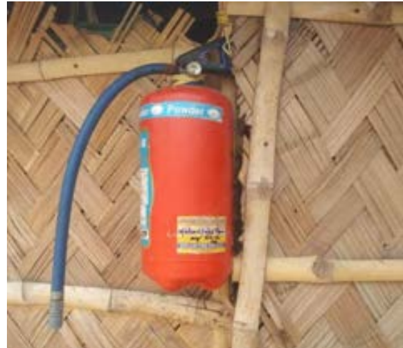
Fig: Replaced fire extinguisher at zone 9 – OHR Bhanagar-II block
