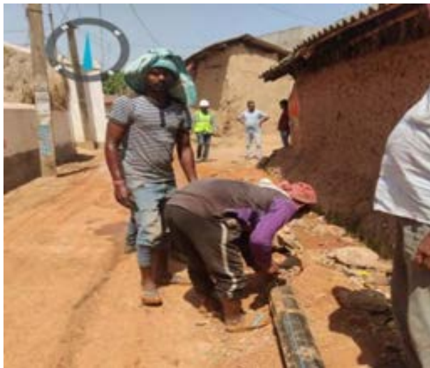
Before: No use of PPEs and incomplete barricading beside the road at HDD site (Package BK/02B)
