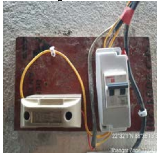
Fig: Proper electrical connection at zone 11-OHR Bhanagar-II block
