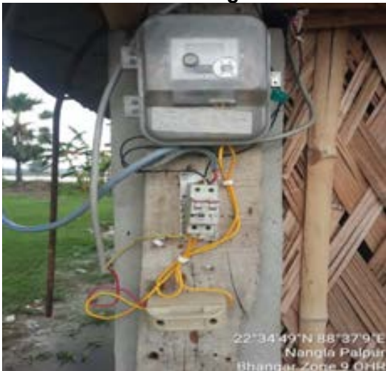
Fig: Damage main switch at zone 9-OHR Bhanagar-II block
