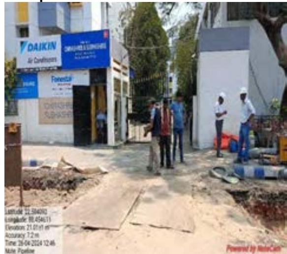
Fig: Metal platform for access to residential complex at street no- 70 Pipeline laying area
