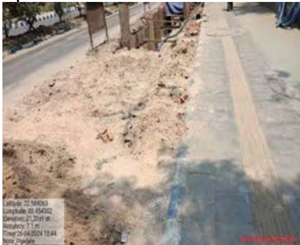
Fig: No platform at street no -70 Pipeline work area
