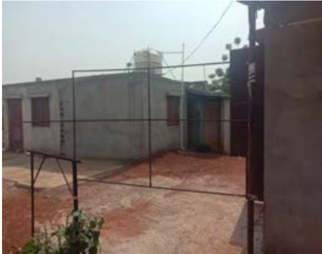
Before: Observed at BK/01 there is no project information board.
