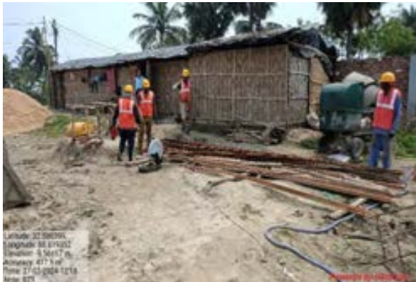
Fig: Zone 9 Pipeline – Use of PPEs during rod binding work at Bhangar-II Block
