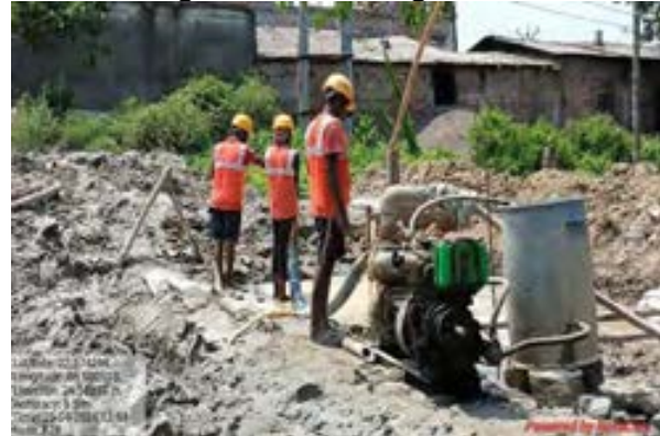
Fig: Zone 8 OHR – Partial use of PPEs during piling work- at Bhangar-II Block
