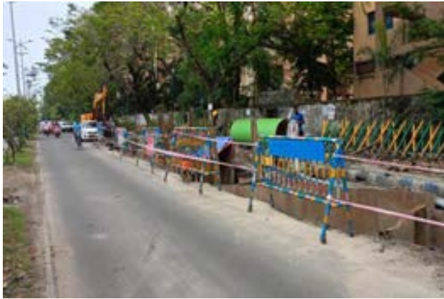
Pipe laying placement of Barricade and caution tape In Street No 71 -WTP
