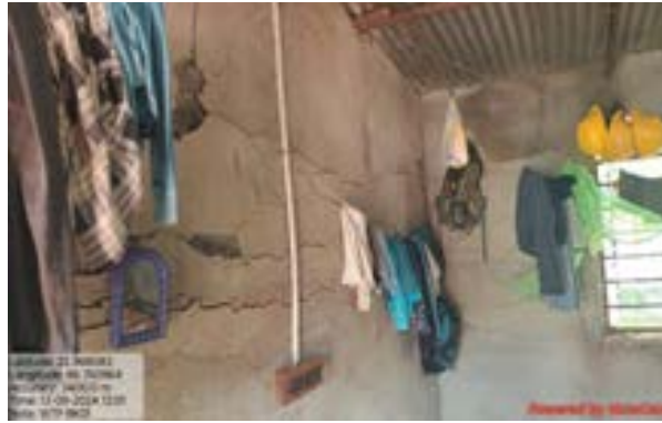
Condition of worker's camp room at intake/ WTP site (package BK/01) needs to be improved
