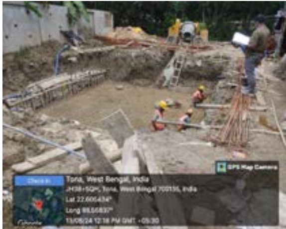
Fig: Zone 5 Pipeline – Use of Partial PPEs in SCADA building construction work-Bhangar II Block
