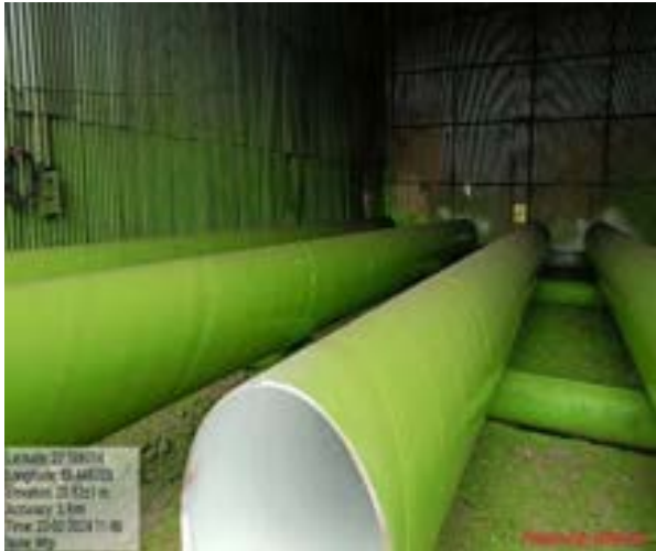
Fig: Spray painting without proper flooring
