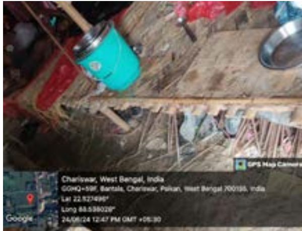
Fig: Zone 3 OHR- Housekeeping is very poor in camp at Bhargar-II Block.
