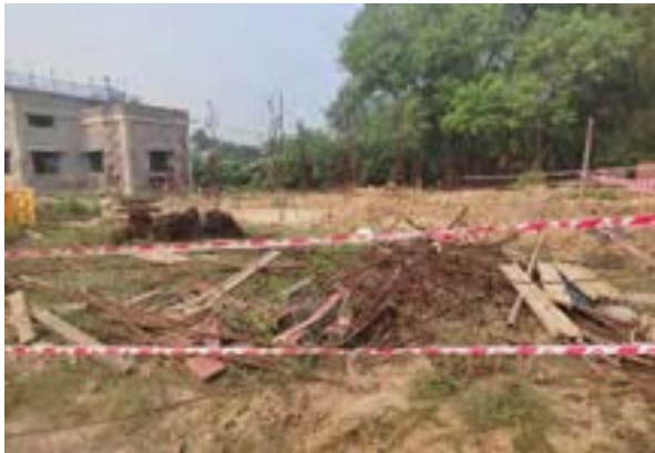
Before: Construction material was scattered condition at site. (package BK/2A)
