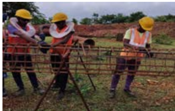
After- Immediately arrangement of proper PPEs for all workers at work site- noted
