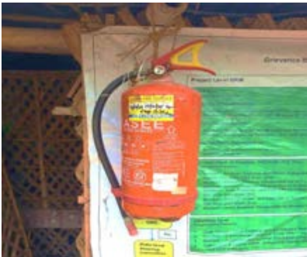
Fig: Filled fire extinguisher in camp area at Zone 5 OHR – Bhanagr-II block
