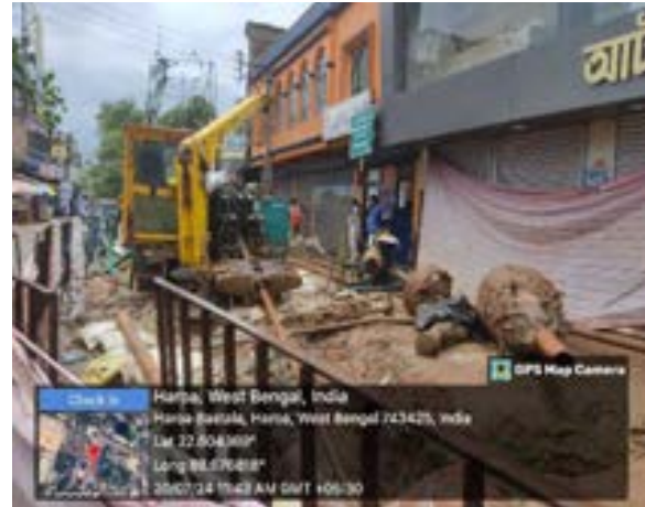
Fig: No platform at working site for the shopkeeper.
