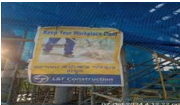
Observed insufficient number of display board BK/2B
