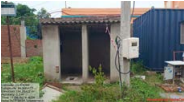
There is no door available on the toilet at Sirmonipur (package BK/2A)
