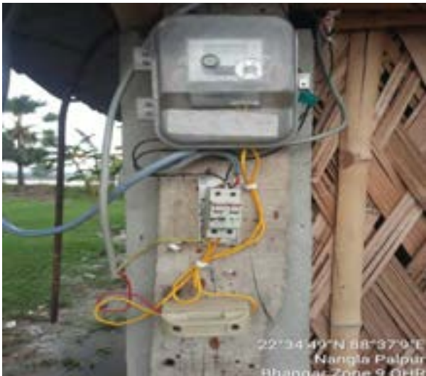
Fig:Damage main switch at zone 9-OHR Bhangar-II block
