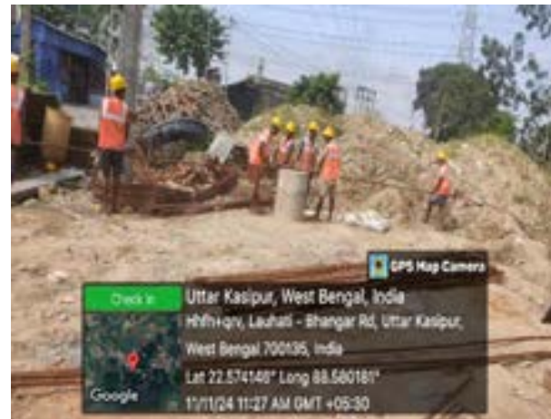
Fig: Zone 8 OHR – Working with partial PPEs in steel setting for OHR construction work-Bhangar-II Block
