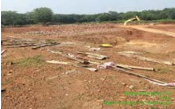
Before: Observed at BK/01 there is no barricade near the excavated area.
