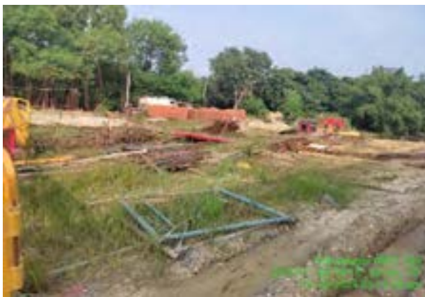
Before: Observed that there was no demarcated scrap yard (Package BK/02A)
