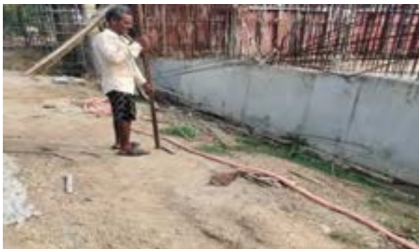
Before- Worker was observed without proper PPE at BK/01
