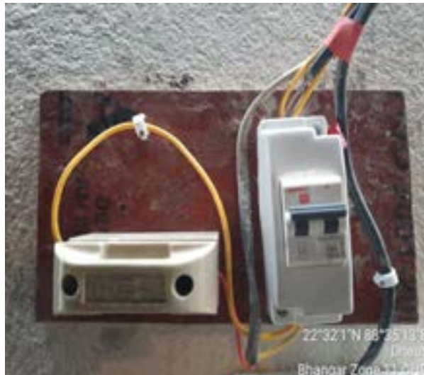
Fig: Proper electrical connection at zone 11-OHR Bhangar-II block
