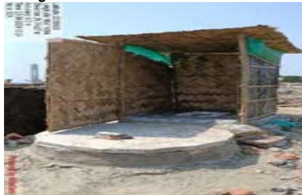
Fig: Twin pit toilet at zone 9 OHR Bhangar-II block
