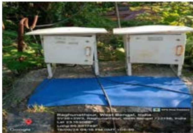
Proper use of rubber mat near electrical DB box (Bk/02A)
