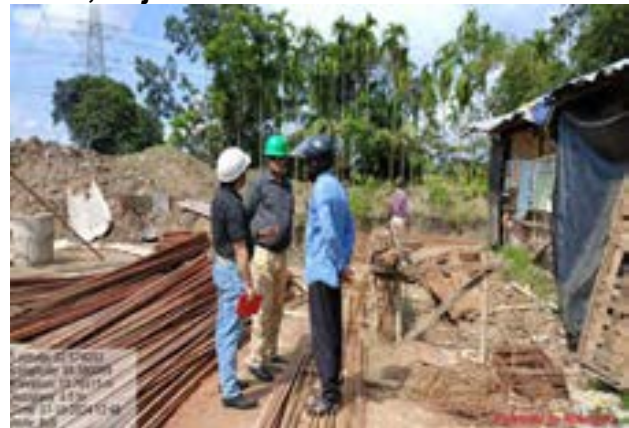
DSISC & PMC representatives discussing with safety officer of contractor, Bhangar II block
