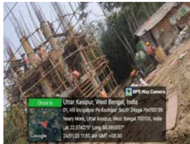
Fig: Zone 8 OHSR – Working with partial PPEs in casting work at OHSR construction - Bhangar-II Block
