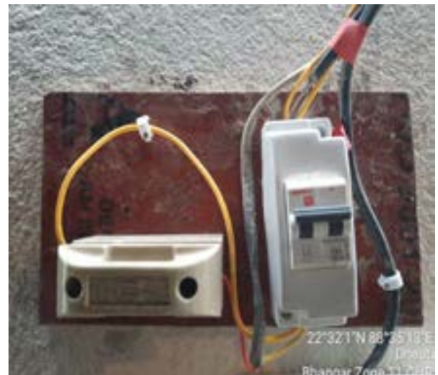
Fig: Proper electrical connection at zone 3-OHR Bhangar-II block
