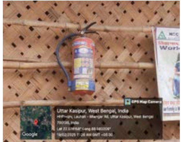
Fig: Replaced fire extinguisher at zone 8 – OHR Bhangar-II block
