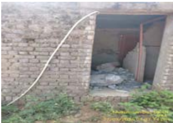
Condition of worker's toilet at intake/ WTP site(package BK/01) needs to be improved.
