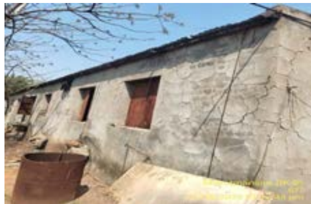
Labour camp is in same condition for the long time, needs to be improve immediately.
