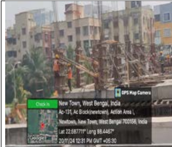
Fig: Partial use of PPEs in WTP site
