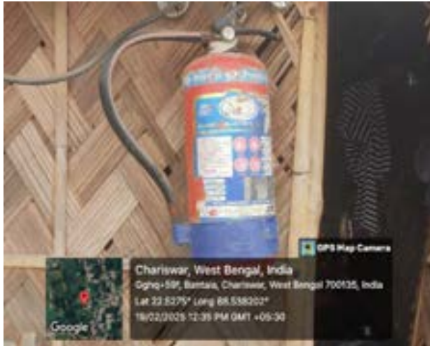
Fig: Filled fire extinguisher in camp area at Zone 3 OHR – Bhanagr-II block
