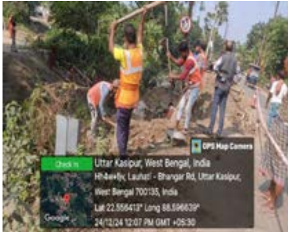
Fig: Zone 8 Pipeline – Use of Partial PPEs in pipe laying work-Bhangar II Block
