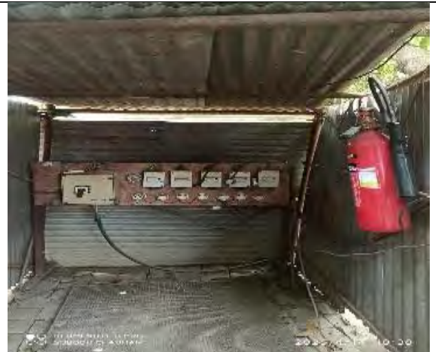
Fig: Partially Complied of electrical safety at BS1 Pumping station
