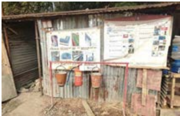
Before: Fire extinguisher near the construction area (Package BK/02A)
