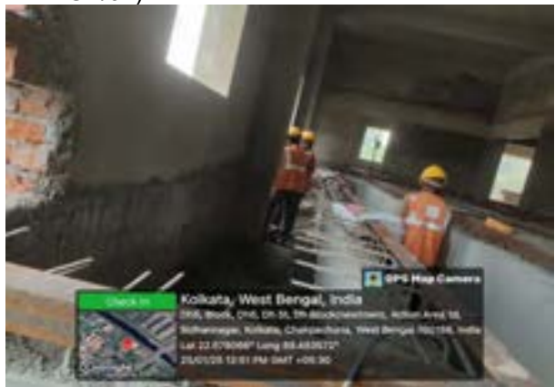
Cable trench activity on going at substation of BS 1 site. (PACK N24PGS/01)
