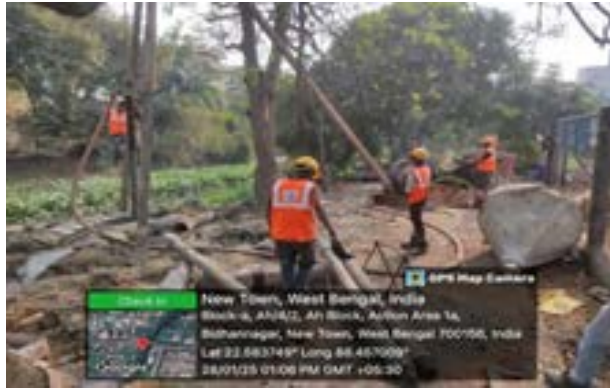
Piling Work is in Progress at Link Canal Crossing Bridge at New Town, Rajarhat. (PACK N24PGS/01)
