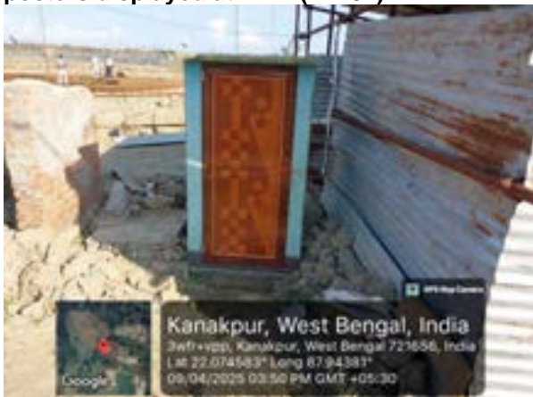
Toilets and washroom available for the workers at Kanakpur OHSR Site
