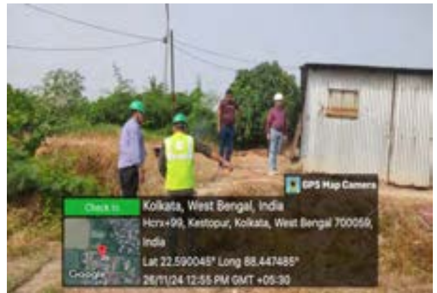
Environment specialist of DSISC, PMC Contractor representatives checked the safety arrangement at work place (PACK N24PGS/01)
