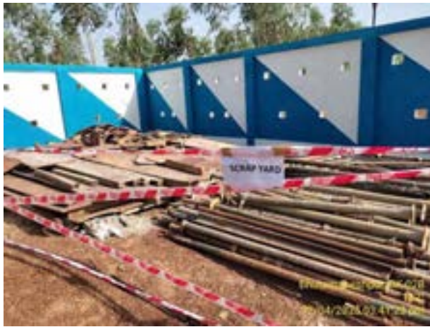
Scrap yard properly maintained Pack Bk/02B
