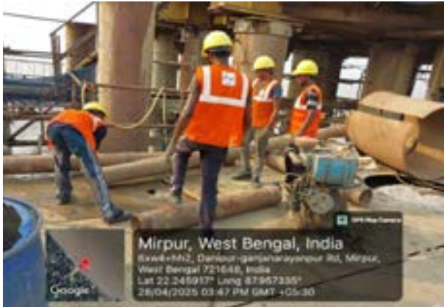
Environmental safety measures at Intake (EM 01)
