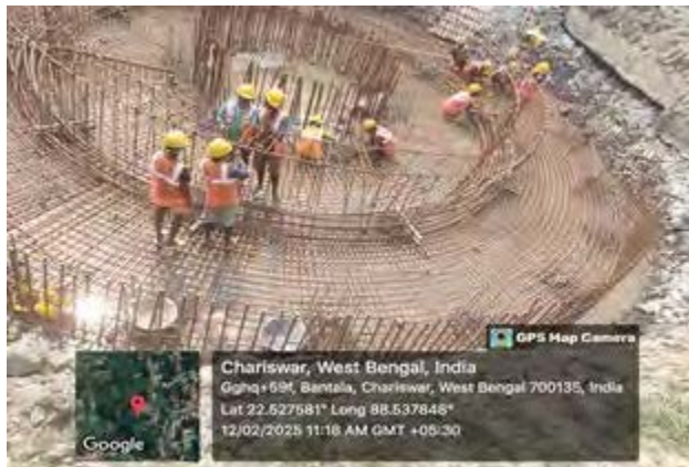
Reinforcement work for OHR foundation is in progress at Zone 3, Bhangar II.(Pack N24pgs/02B)
