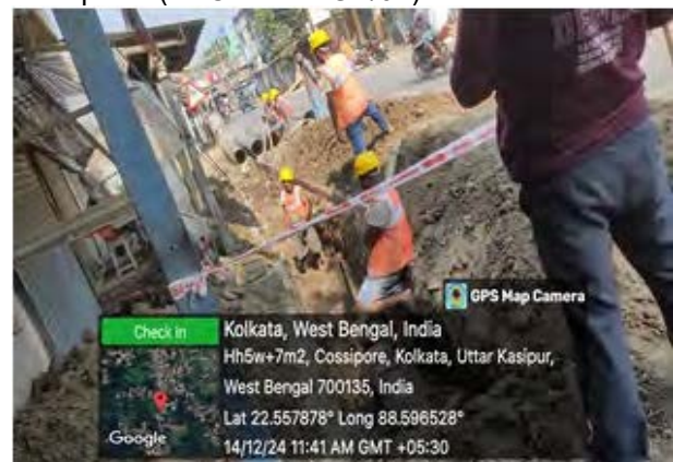
The laborers are engaged in laying 400 mm dia HDD pipe at the Bhangar-Lauhati main road Side. (Pack N24pgs/02B)
