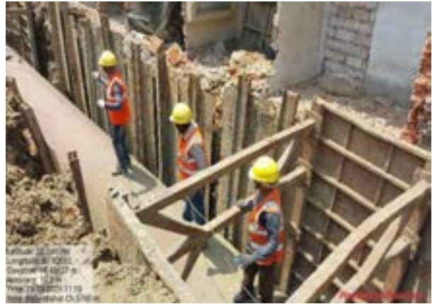
EHS Compliance: Safety precautions taken during 1400 dia. RWTM MS pipe laying work near Byabattarhat (SH 4) (EM 01)
