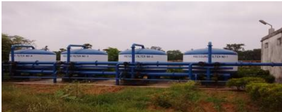
Pressure Filters at the Gangajalghati WTP
