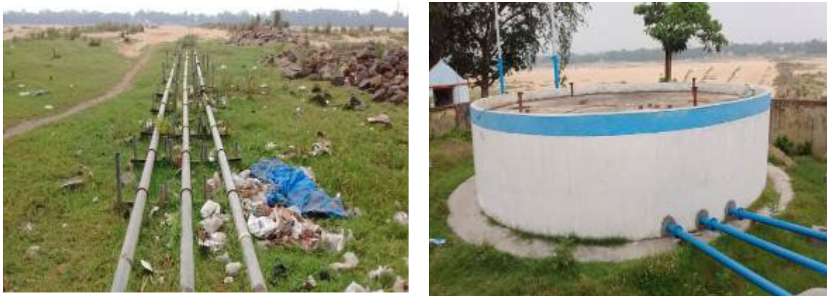
Raw water mains from river bed tube wells and the new reservoir
